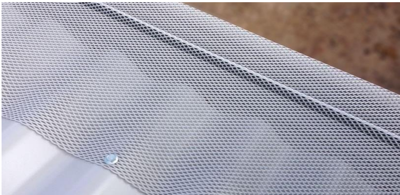
Figure 1.1 - Standard GPS Ember Guard installed on Corrugated roof.
